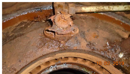
Main Engine cooling Water connection & exhaust valve seat bores
