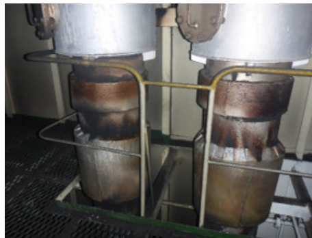
Exhaust Leakage at AE Update
