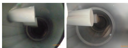
Main Engine Exhaust Manifold
