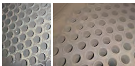
Exhaust gas Boiler tubes
