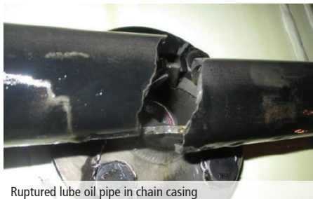
Ruptured lube oil pipe in chain casing
