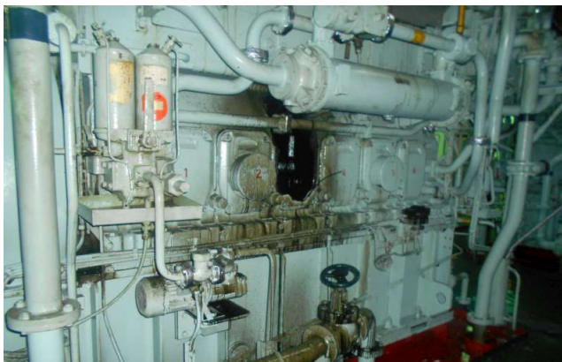
Damaged engine frame in way of unit #3 crank case
