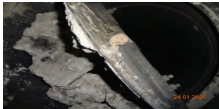
Deposits in the exhaust pipeline and valves
