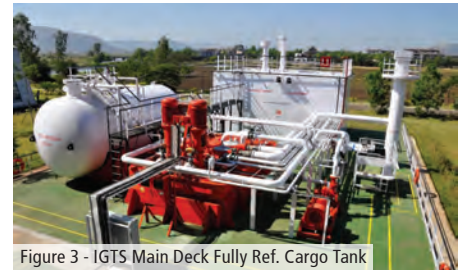
Figure 3 - IGTS Main Deck Fully Ref. Cargo Tank
