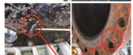
Small groove allowed oil leak
